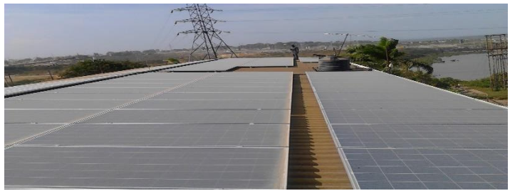
Figure 8: The 40 KW Grid-tied solar at Kipevu- Thermal Region.
