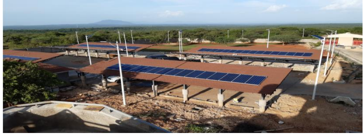
Figure 7: The 30 KW Grid-tie solar at Hydro Plaza- Easter Region.
