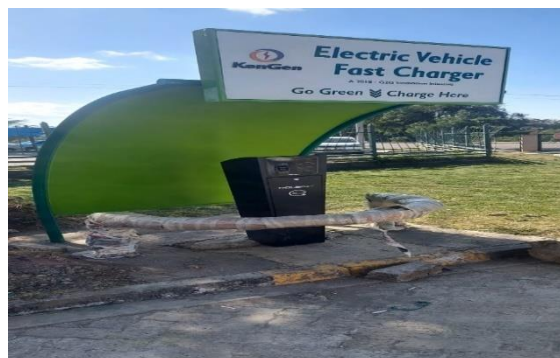
Figure 12: Geothermal Plaza EV Charger.
